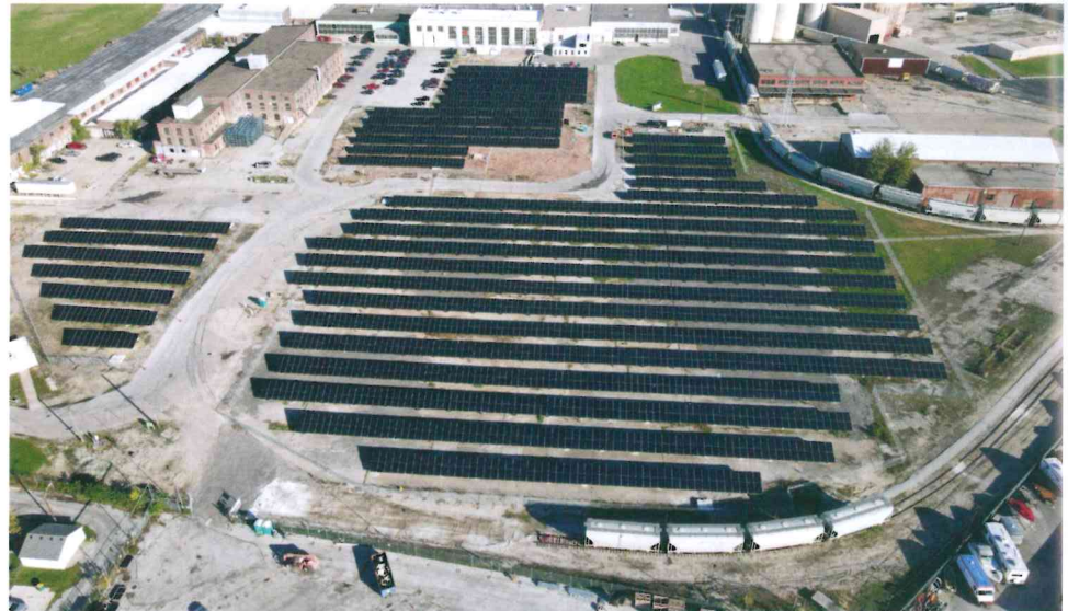
A solar array nearing completion at the NSG Group facility in Rossford, Ohio. The 1.4MW solar array installation, using NSG Group's solar energy glass products, is being constructed by AEP OnSite Partners, an affiliate of American Electric Power. According to the NSG Group, the solar array will supply about 2.5 million kWh of renewable energy annually. Photograph courtesy of NSG Group, 20 October 2021.
