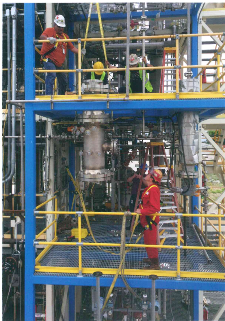
SwRI specializes in developing new processes for creating hydrogen and other fuels. We then demonstrate these processes in pilot plant facilities (shown here) that can be scaled up for actual production plants.
