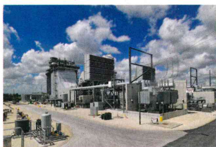
3. GE 7HA.03 gas turbine unit installed at Florida Power & Light's Dania Beach Clean Energy Center in Florida can run blends of up to 50% hydrogen and natural gas. Courtesy: GE Gas Power
