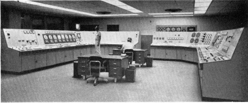
Fig. 3.—Control Room, Tijeras.
