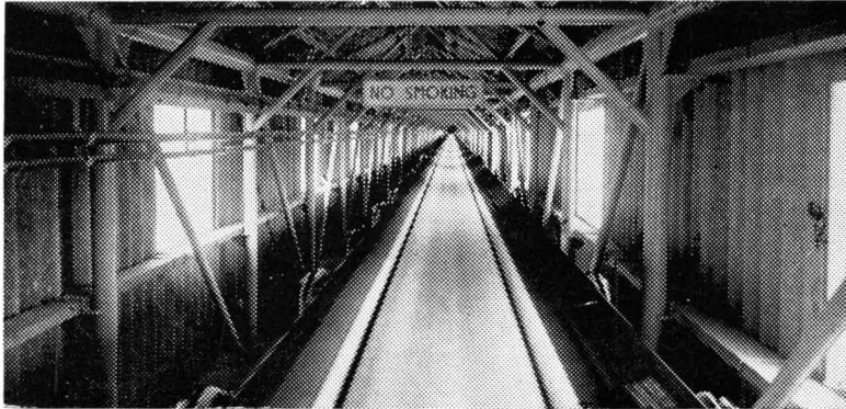
A Typical BARRY Troughed Belt Conveyor in a Tubular Gantry
