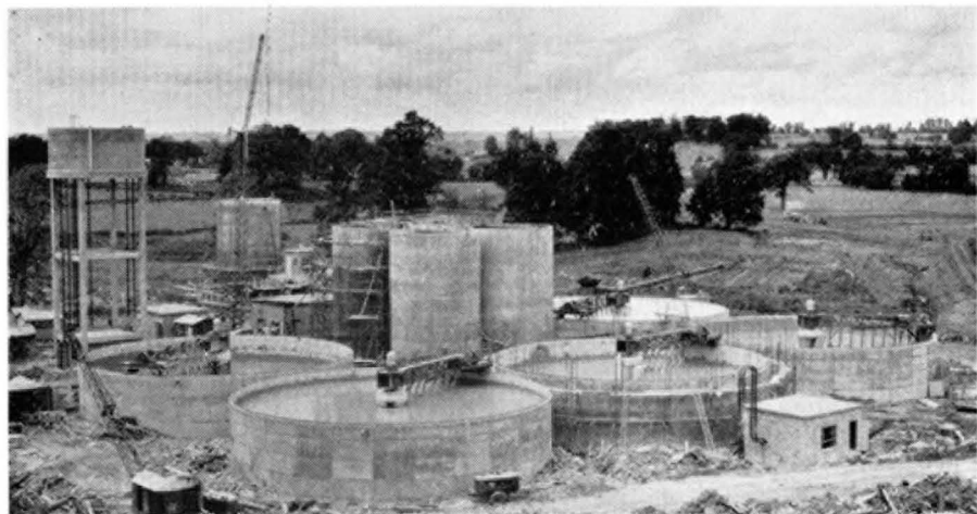
Fig. 6.—Slurry Doctor and Storage Tanks.
