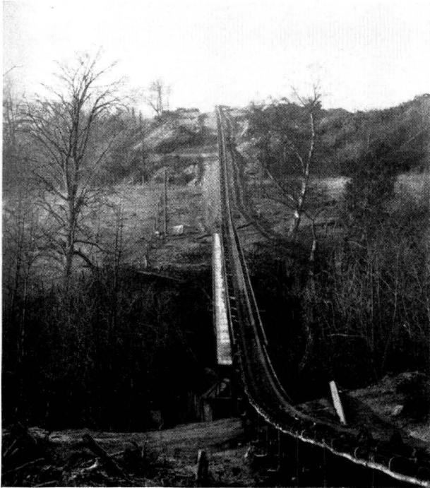
▲ Meco Suspended Idler Belt Conveyor with a 155 ft. bridge crossing a wooded valley.
