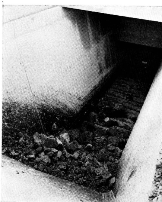
Fig. 5. Grizzly Feeder at Southam Works.
