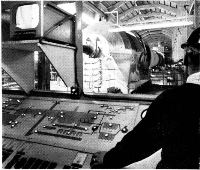
Fig. 16. Control Panel and Firing End of Kiln.
