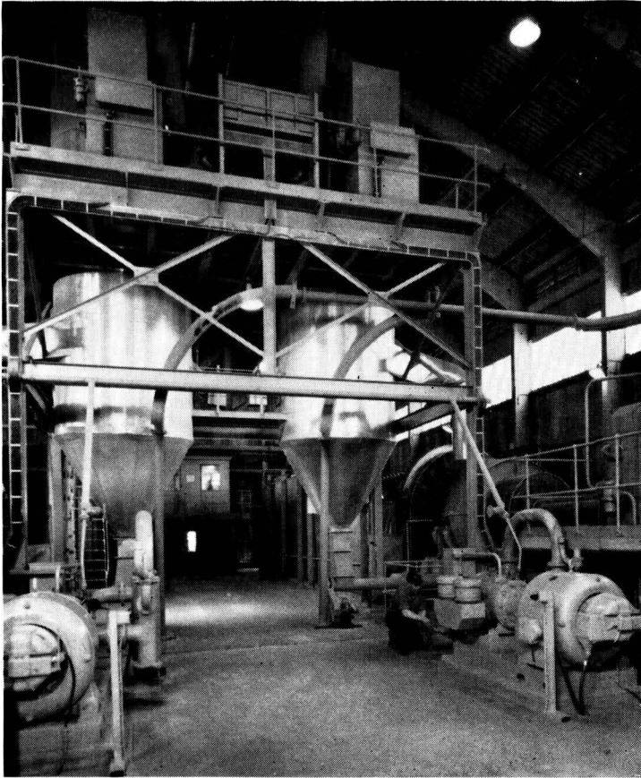
Fig. 22.—Electrostatic Precipitators at Cement Grinding Mills.
