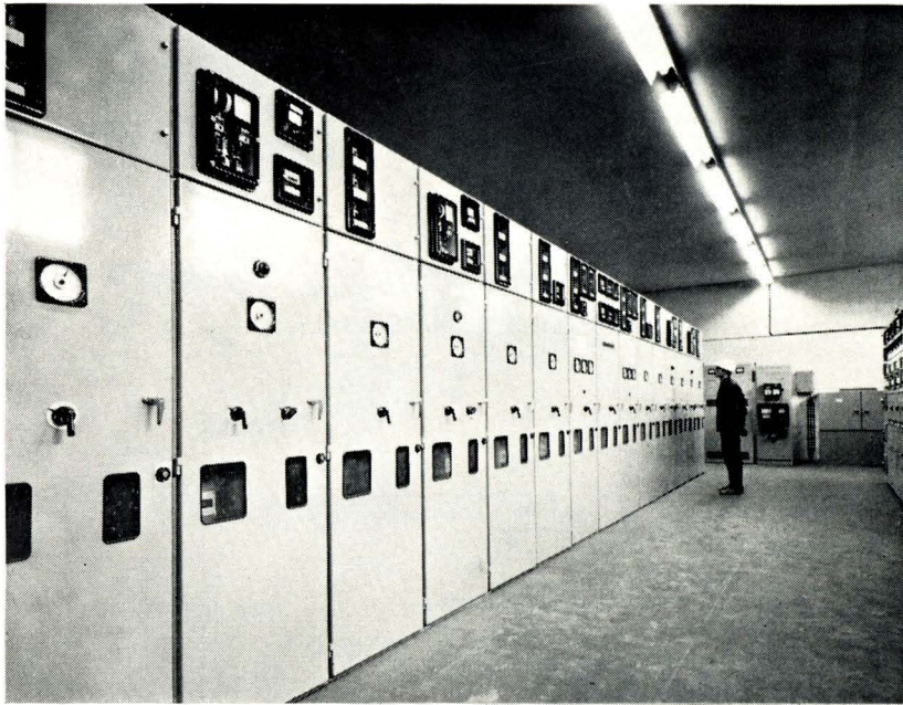
Fig. 26.—Works Main Substation.
