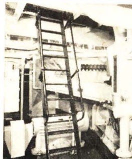
Fuller Kinyon pump with F-H Airslide conveyors from fluid lift.
