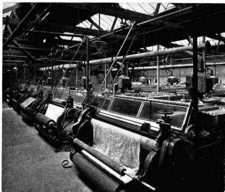
Hooding and Vapour Collecting Ducts in a British Rubber-proofing Works.
