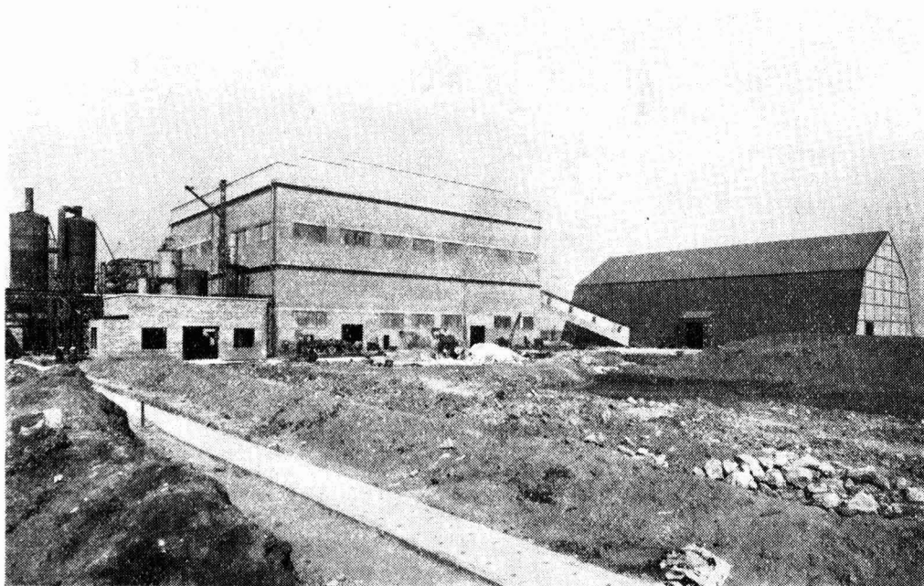
General view of the acid plant, showing storage silo, main building and external conversion plant under construction
