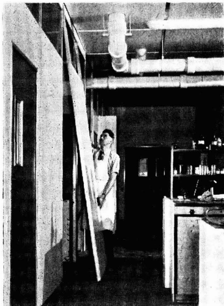
Fitting one of the demountable 'Holoplast' panels, which are fixed at the top by steel brackets connected to the main structure and at the bottom by a screw tapped into the floor
