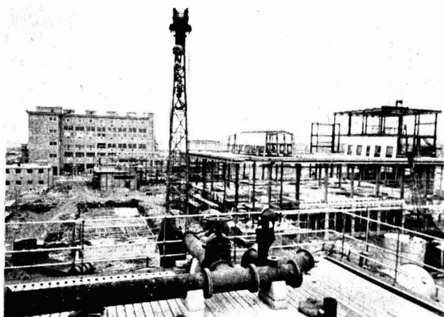
A recent picture showing constructional work in progress on the polymer section of I.C.I.'s 'Terylene' plant at Wilton. The plant was commenced in July, 1952, and since then work has proceeded day and night and is up to schedule. The first unit of this £20,000,000 project will be completed by the end of this year
