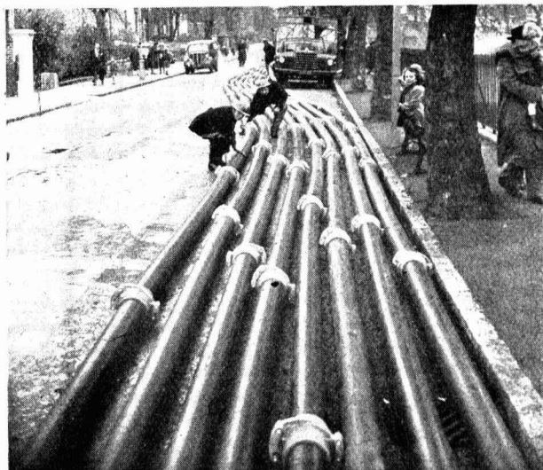
A water-relaying exercise, using 6-inch polythene piping, was carried out recently in London by 400 members of the Auxiliary Fire Service. The piping was in 16-foot lengths, weighing 50 pounds each, and officials were impressed with the advantages which the plastic piping has over the same size of rubber hose
