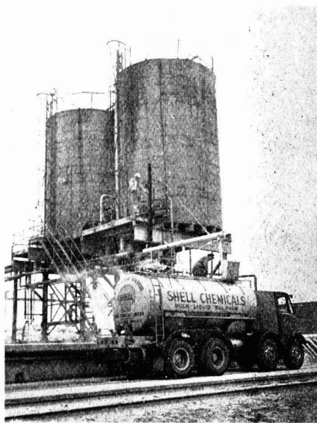
The bulk liquid sulphur installation
