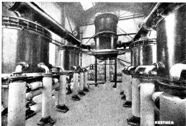
Waste Sulphuric Acid Recovery Plant
