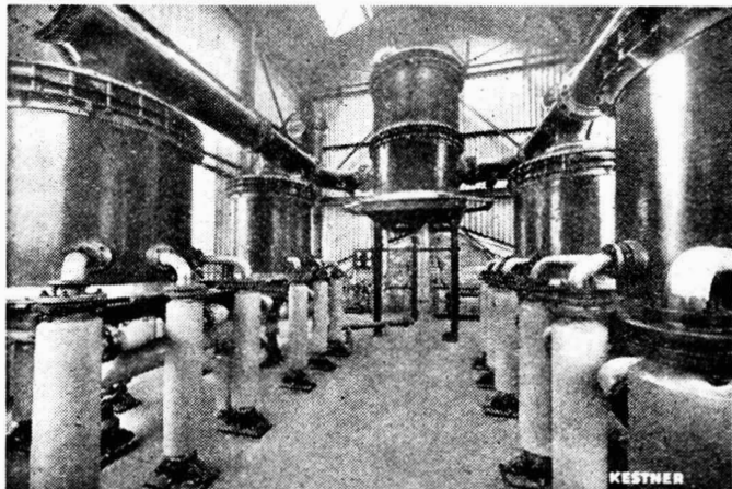
Waste Sulphuric Acid Recovery Plant
