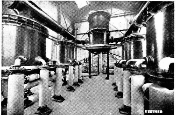
Waste Sulphuric Acid Recovery Plant
