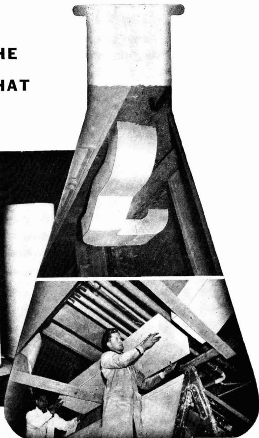
'Darvic' p.v.c. has been installed for fume removal ducting in a new building at the Rothamsted Experimental Station. Contractors: Vent-Axia Ltd., and The Chemical Pipe & Vessel Co. Ltd.
