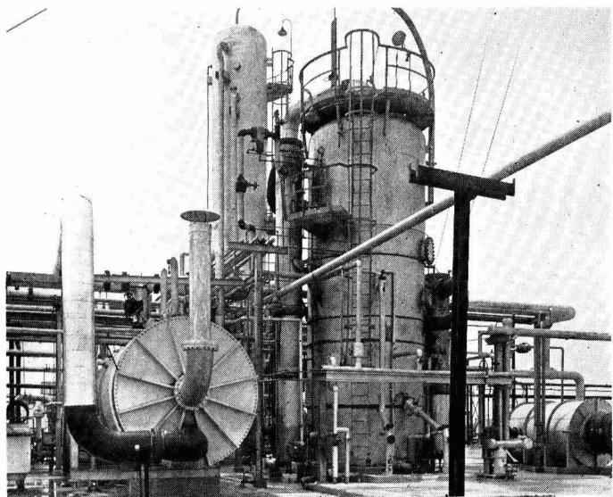
Condenser column and converter unit at Marcus Hook
