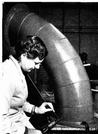
Welding of rigid Vybak p.v.c. ducting made up from sections of extruded tube by Extrudex Ltd., Bracknell. Courtesy Bakelite Ltd.
