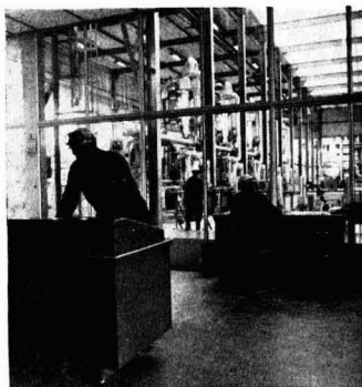
Control room for the copolymerisation unit, for which Matthew Hall were contractors
