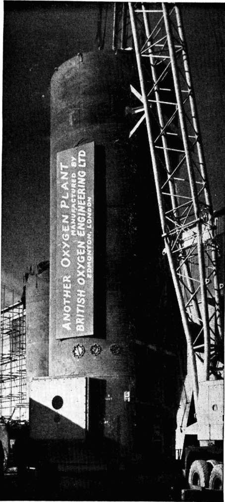
One of the air separation units, weighing 24 tons, is lifted into position.
