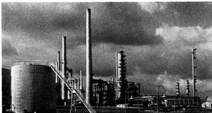
In the background are the crude oil distillation unit, light ends recovery unit and Powerformer.
