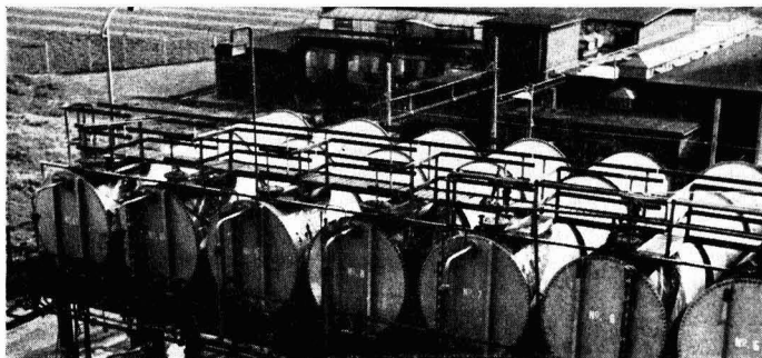
Part of a battery of rubber-lined stock tanks for storage of sodium hypochlorite liquor and hydrochloric acid at Murgatroyd's Salt and Chemical Co. Ltd., Sandbach, Cheshire. Each tank is 30 ft. long and 7 ft. 6 in. in diameter
