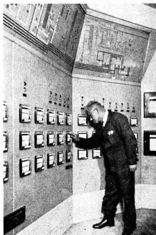
Part of the process flow indicator and recorder panels of Grange Chemicals' detergent alkylate plant at Grangemouth
