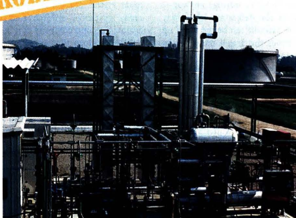
Photo courtesy of Zimpro Environmental Inc.
