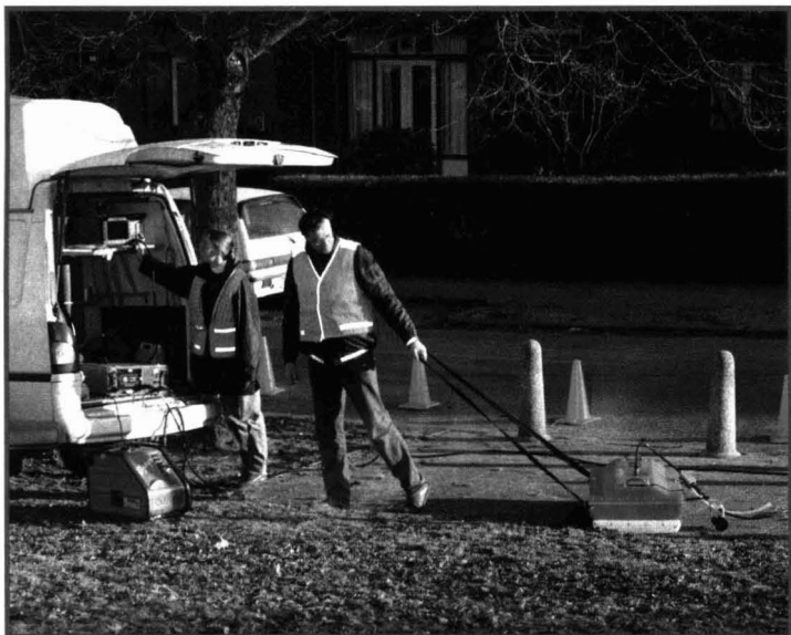
Ground penetrating radar (GPR) locates and defines the extent of hydrocarbon contamination.
