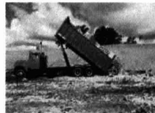
Landfill Gas Analysis
