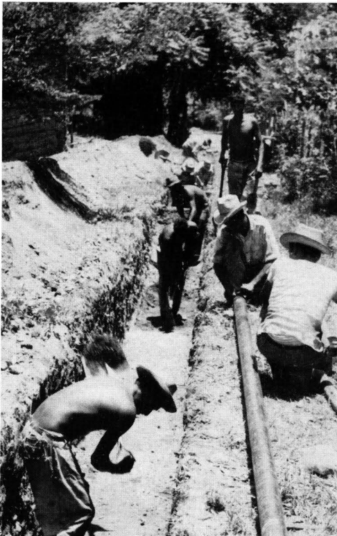
Water mains. To increase the supply of water, villagers lay water mains in the rural village of Poa, State of Yaracuy, Venezuela
