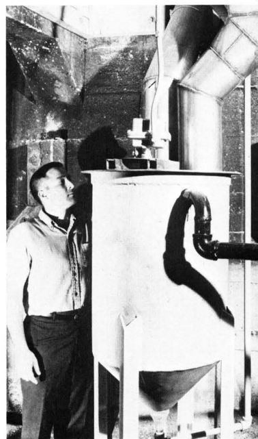
Slurry. View of control panel shows slurry tank and carbon hopper
