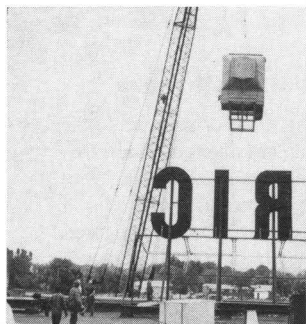
Scrubber unit installed at GE plant
