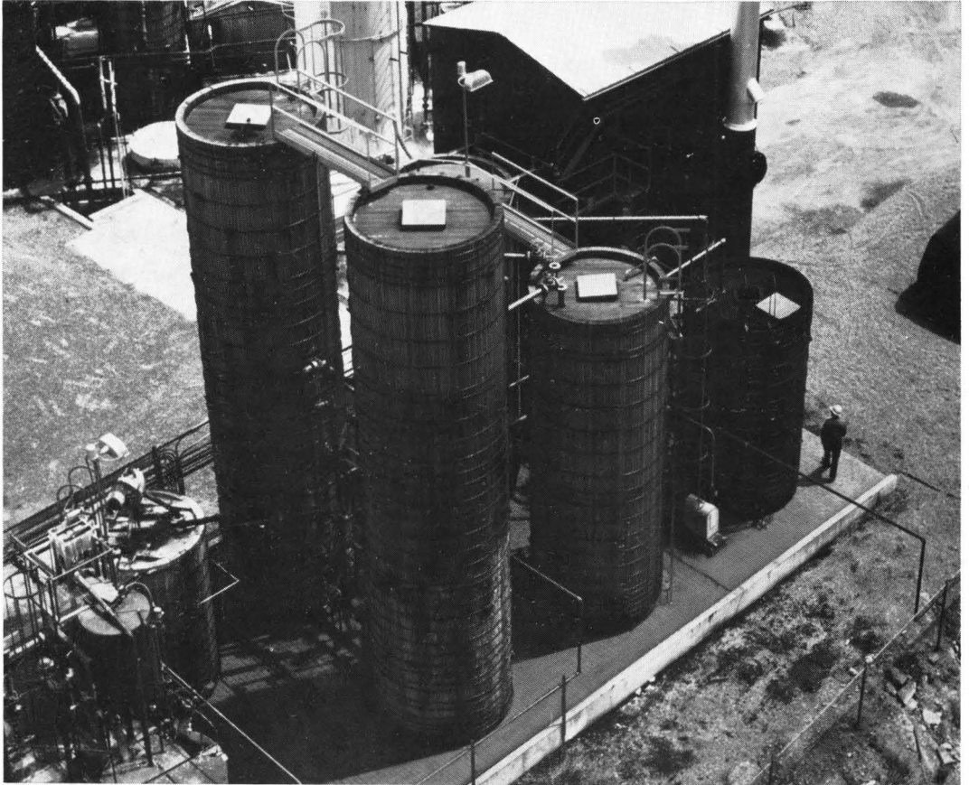
This Filtrasorb System is designed to remove dissolved organic chemicals from 150,000 gallons of wastewater per day. Total land area is only 45 feet by 30 feet.
