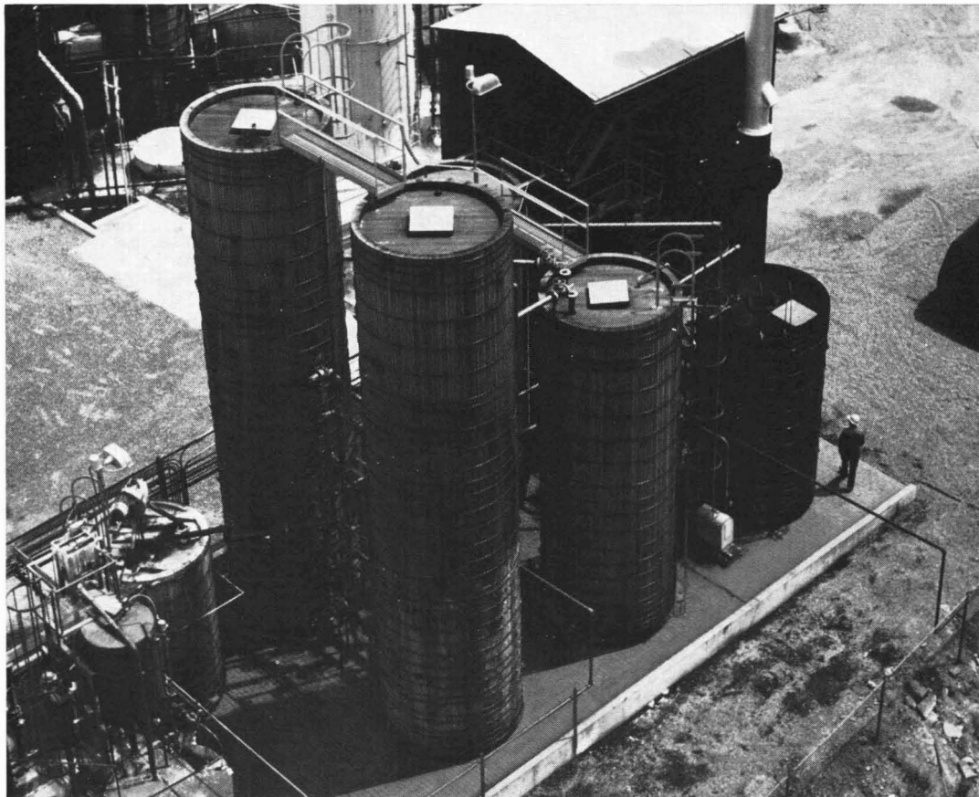
This Filtrasorb System is designed to remove dissolved organic chemicals from 150,000 gallons of wastewater per day. Total land area is only 45 feet by 30 feet.
