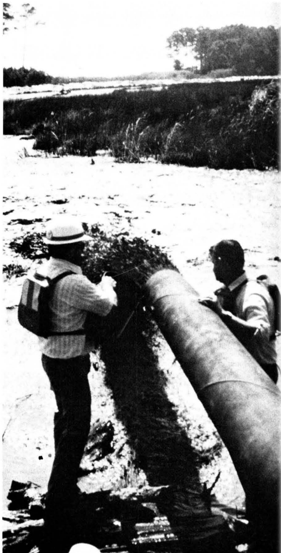
Disposal. Dredged material is in the process of being slurried to a disposal site
