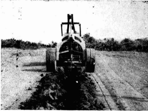
Fig. 2. Slit 2½ ft deep being made (Courtesy Mr. H. N. Parsons, Field Supt., Enmore Estates Ltd.)
