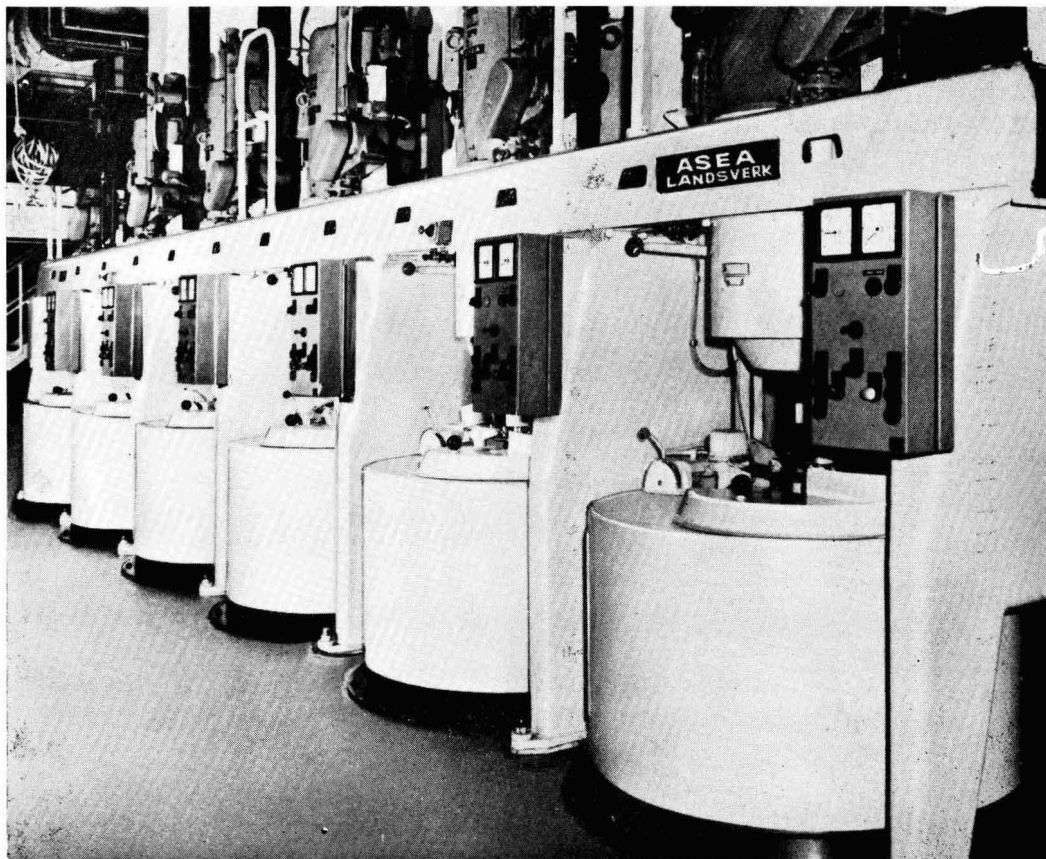
One of the batteries delivered to The Colonial Sugar Refining Co., installed in the Pyrmont Refinery, Sydney.
