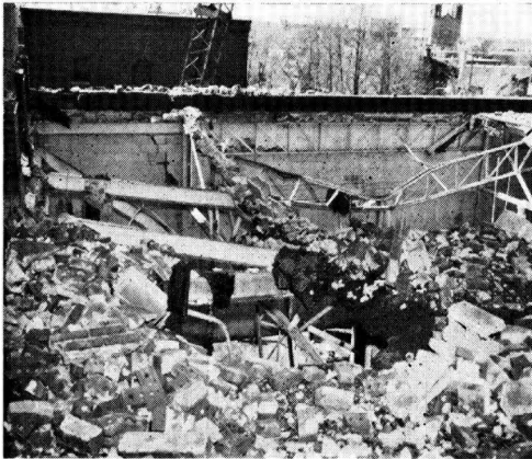
Fig. 3. Damage to the roof of the refined sugar warehouse caused by the east wall of the packing building falling through it.
