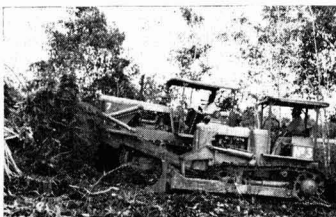
A Fowler Challenger 33 and a Track-Marshall both fitted with Marshall hydraulic angledozers working together to clear bush during extensions to sugar plantations on the Leonora estate of the Demerara Company, Guyana.
