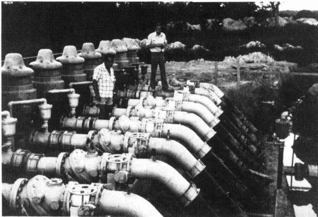
A 75 million gallons/day pumping station for an Ivory Coast cane estate
