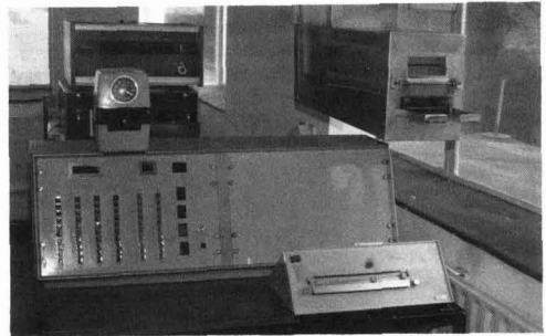
Fig. 2. Ipswich weighbridge installation showing Avery weighbridge electronics in the background, operator's data entry panel and weigh ticket printer in the foreground, and Sorensen document conveyor on the right
