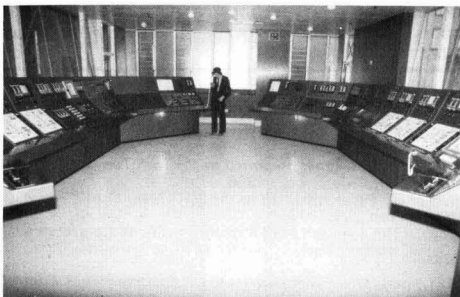
Fig. 7. General view of the Newark sugar end control room
