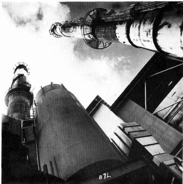
Fig. 5. One of six Ducon fly ash arrestor vessels, Victoria mill
