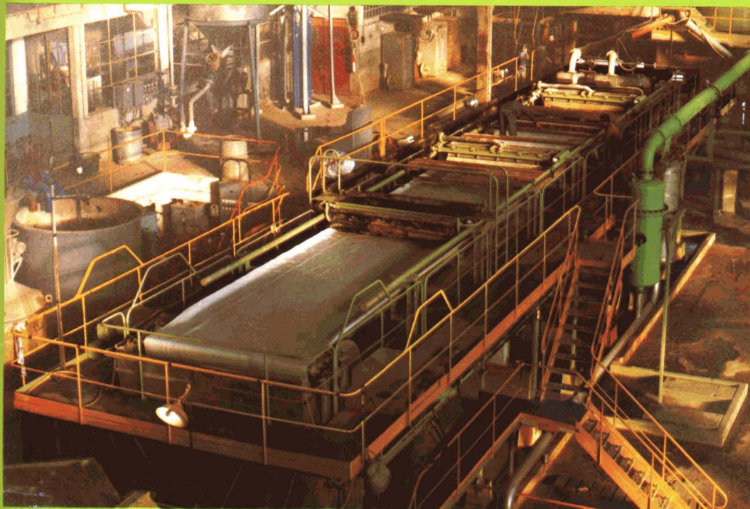
horizontal vacuum belt-filter of 45 m 2 installed at SIMO BESSINES (France)
