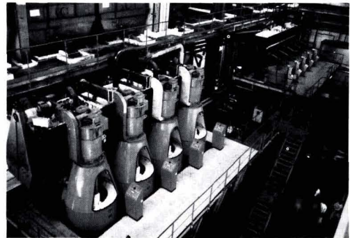
Centrifugal station of the N'Koteng, Cameroons, cane sugar factory. In the foreground, four "COMPACT 411" centrifugals. In the background, five continuous "FC 1000" centrifugals.
