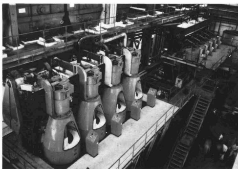
Centrifugal station of the N'Koteng, Cameroons, cane sugar factory. In the foreground, four "COMPACT 411" centrifugals. In the background, five continuous "FC 1000" centrifugals.
