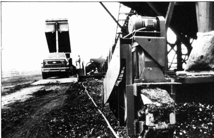
Fig. 4. Individual electric motors and Link-Belt speed reducers drive the tracks that move the piler back to start another pass and build the pile of beets
