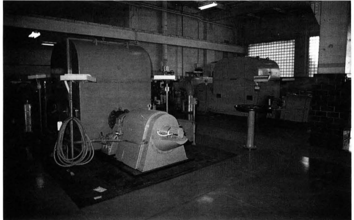
Turbogenerators for supplying power to the refinery
