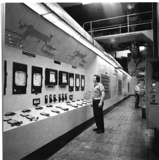
Figure 3. A control room Tate & Lyle's Thames refinery
