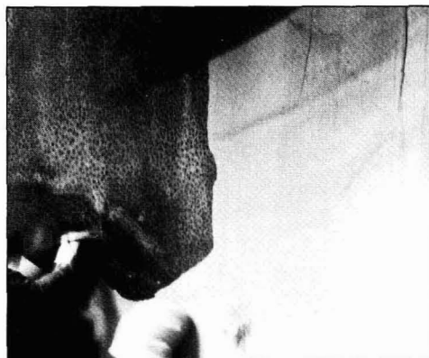
Figure 3—In the third stage of corrosion, the polyester lining has lost adhesion. Spot corrosion or rusting appears beneath the coating
