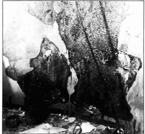
Figure 5 —In the fifth stage of corrosion, considerable loss of steel and delamination has occurred. A small hole completely thru liner permits the corrosive media to attack both front and back surfaces of the steel liner
