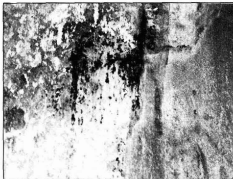
Figure 2—In the second stage of corrosion, black iron oxide or iron sulfide appears thru weakened lining
