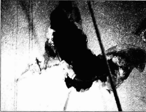
Figure 6—Final stage of corrosion causes a hole about 1 ft × 2 ft thru the ¼" thick A-242 type steel. A plate will be welded over this area and new lining applied
