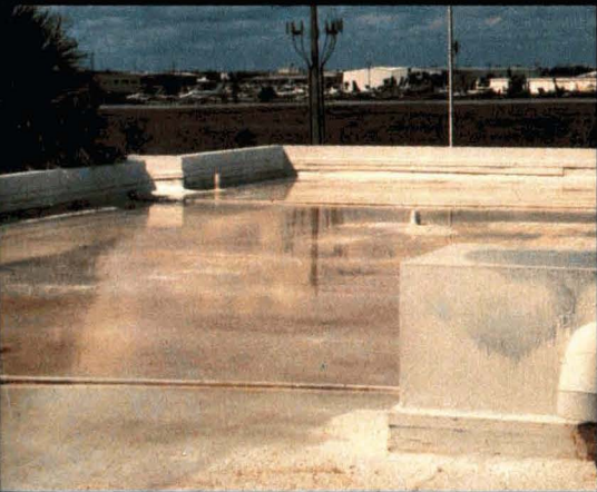
This roof in Florida demonstrates how a roof mastic based on RHOPLEX EC-1895 acrylic retains its initial integrity under ponded water conditions.
