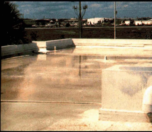
This roof in Florida demonstrates how a roof mastic based on RHOPLEX EC-1895 acrylic retains its initial integrity under ponded water conditions.
